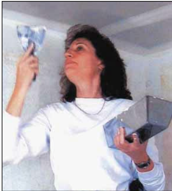
Pamala Anderson, owner of Anderson Construction in Greencastle, works on a ceiling in one of her homes she's remodeling in Chambersburg.
